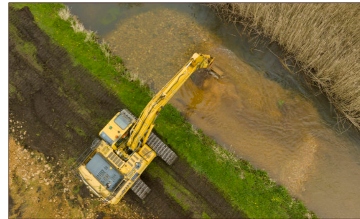
Top: The 360 is able to deposit stone and gravel to about ¾ of the way across the channel from pre-delivered piles arranged along the bank. This minimises damage from the digger and speeds up the process.
